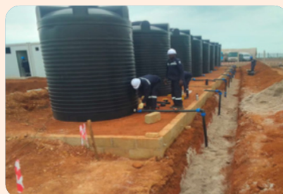
Domestic water supply connection for storage tanks
