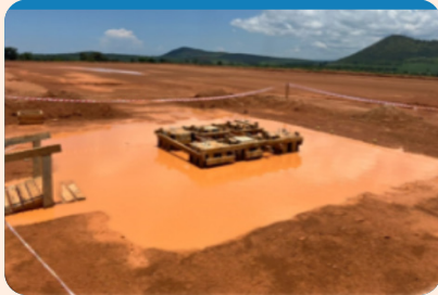
Corrosion inhibitor tank foundation
