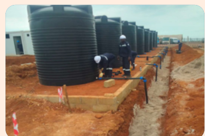
Domestic water supply connection for storage tanks
