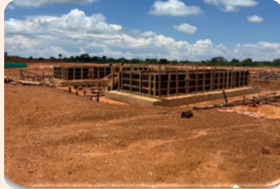
Export pump foundation
