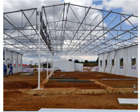
MCPY-15 CTR Canteen installation
