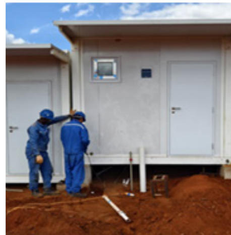
VIP Roomm Pipe connection
