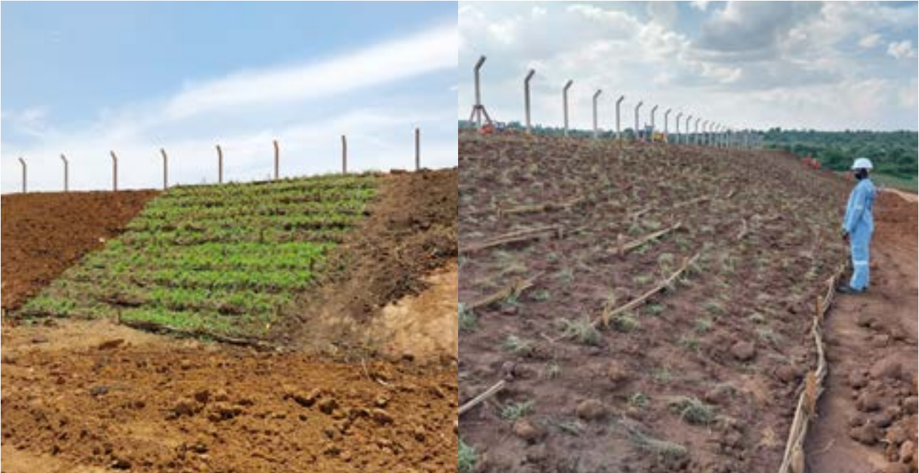
Figure 11: Growing of grass on the slopes at MCPY03 to promote slope stability
